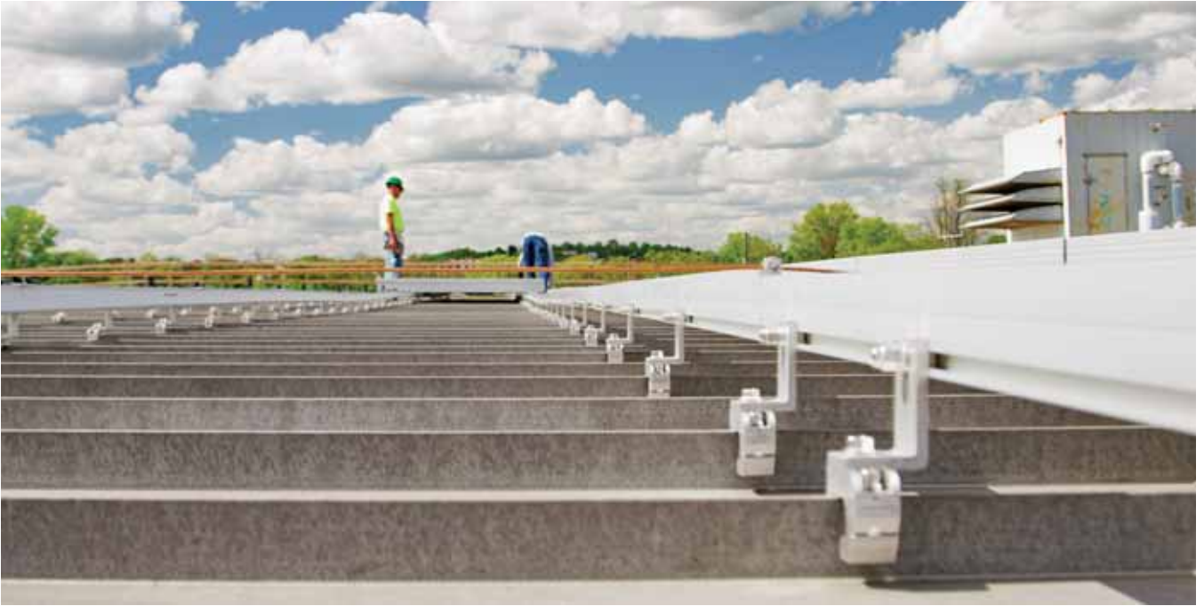
Systems installed on low-sloped metal roofs may be more affected by high snow loads. Be sure to follow the local codes for wind uplift and snow loading for whatever the roof slope is.
